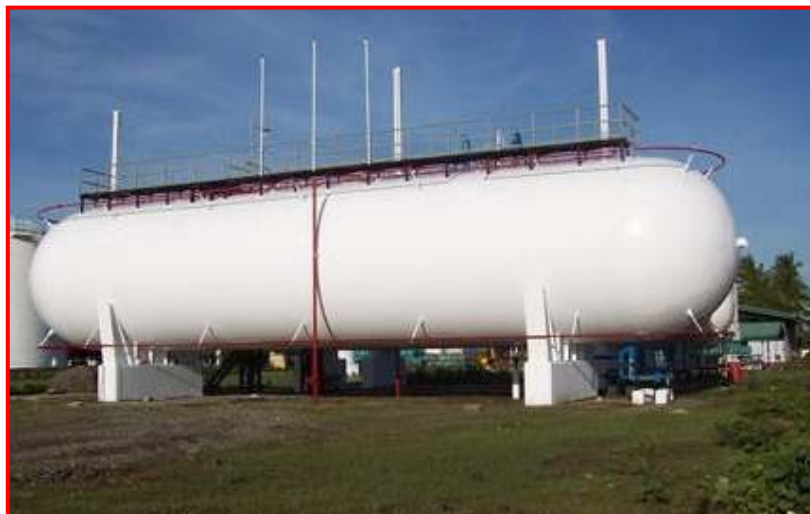
Gas Bullet Tank Installation
