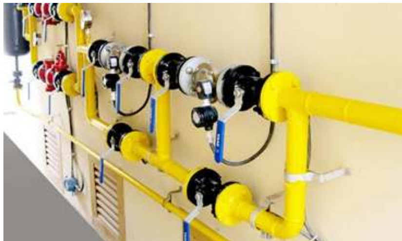
LPG Reticulation System (Pipe Gas System)
